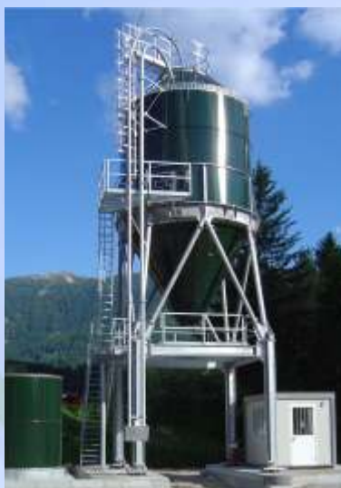
Silo for salt 240t Monteciaro, Italy
